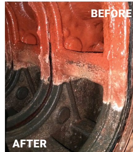
Upper steam chest in cast iron boiler.
